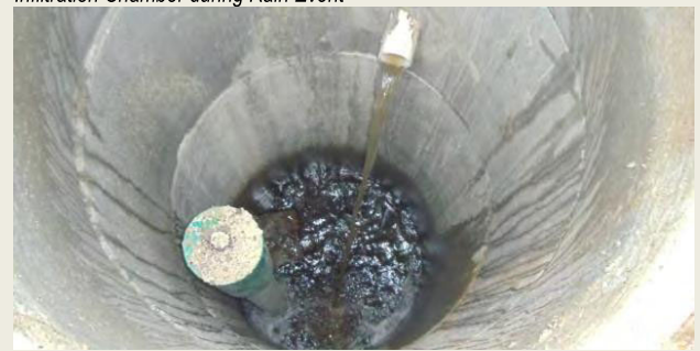
Infiltration Chamber during Rain Event
