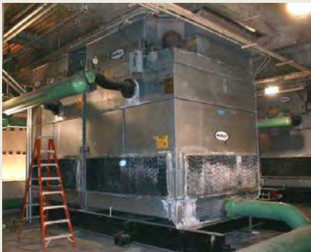
Evaporative Condenser (note scale buildup on front right)
