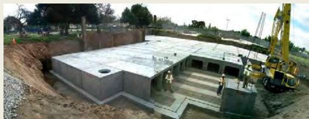
Underground infiltration gallery in Garvanza Park
