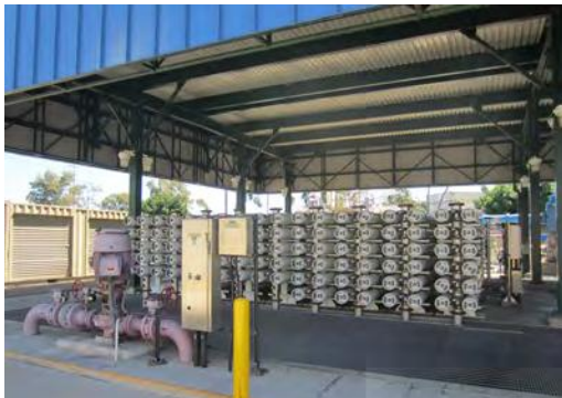
Terminal Island Water Reclamation Plant
