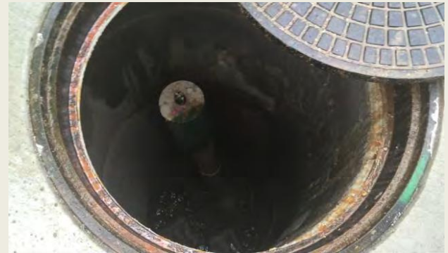
Infiltration Chamber during Rain Event
